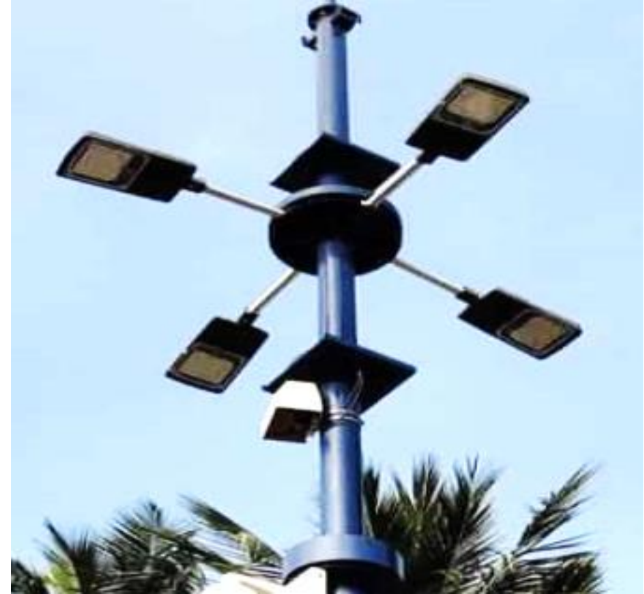
Multipurpose Smart Pole , Chennai
