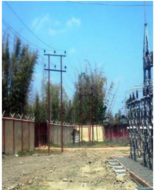
33 kV (H Pole) line inside substation
